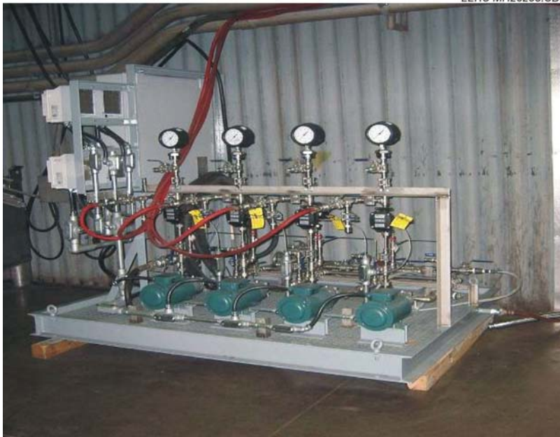
Figure 3. Photograph of a skid used to spray additives onto the coal.
